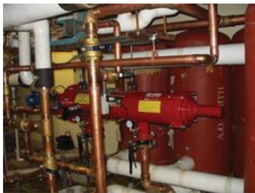
The installed filter is "green technology."
