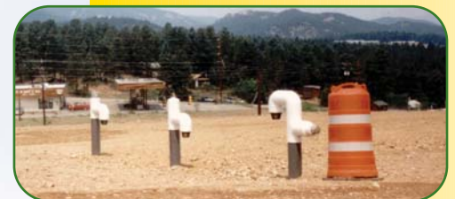
3-Tank System with above ground filters, connections and manway access.
